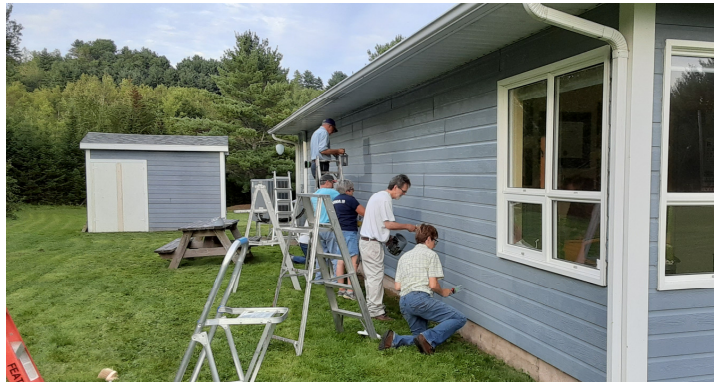
Volunteers from communities around the area have completed painting the exterior of the New Germany & Area Medical Centre. Thank you to all involved.
